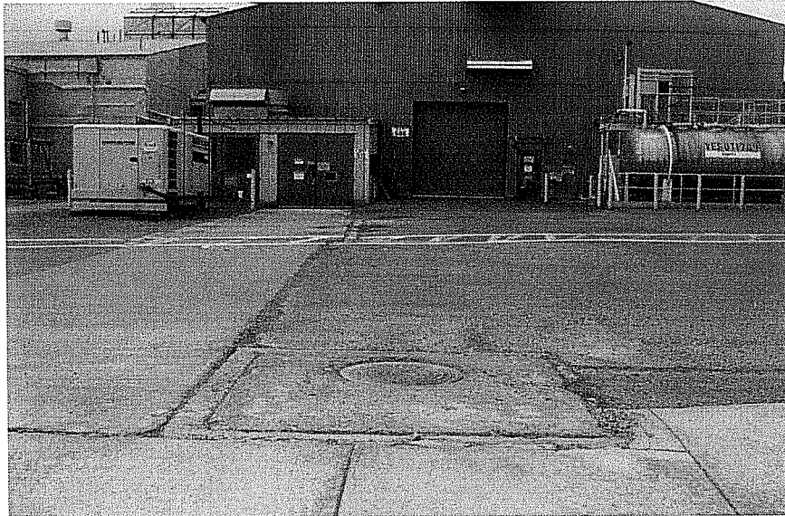
Figure 1. Photograph showing a portion of Beech Street and the cover to Manhole MAH-PHE-291.
