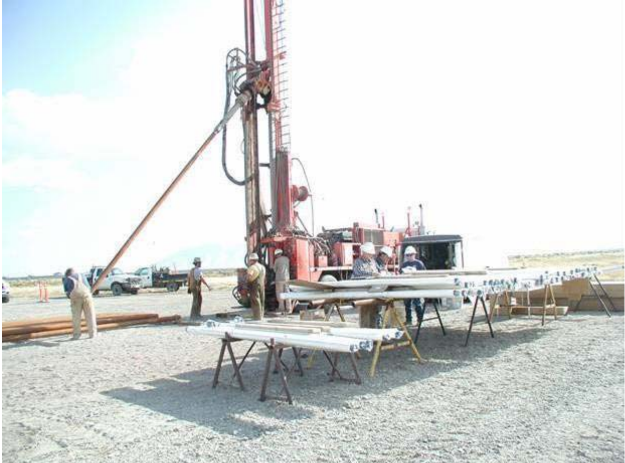
Figure D-1. Major's dual-rotary drill rig (Foremost DR-24) and accessory equipment used for installing the Westbay Packer System at MIDDLE-2051.
