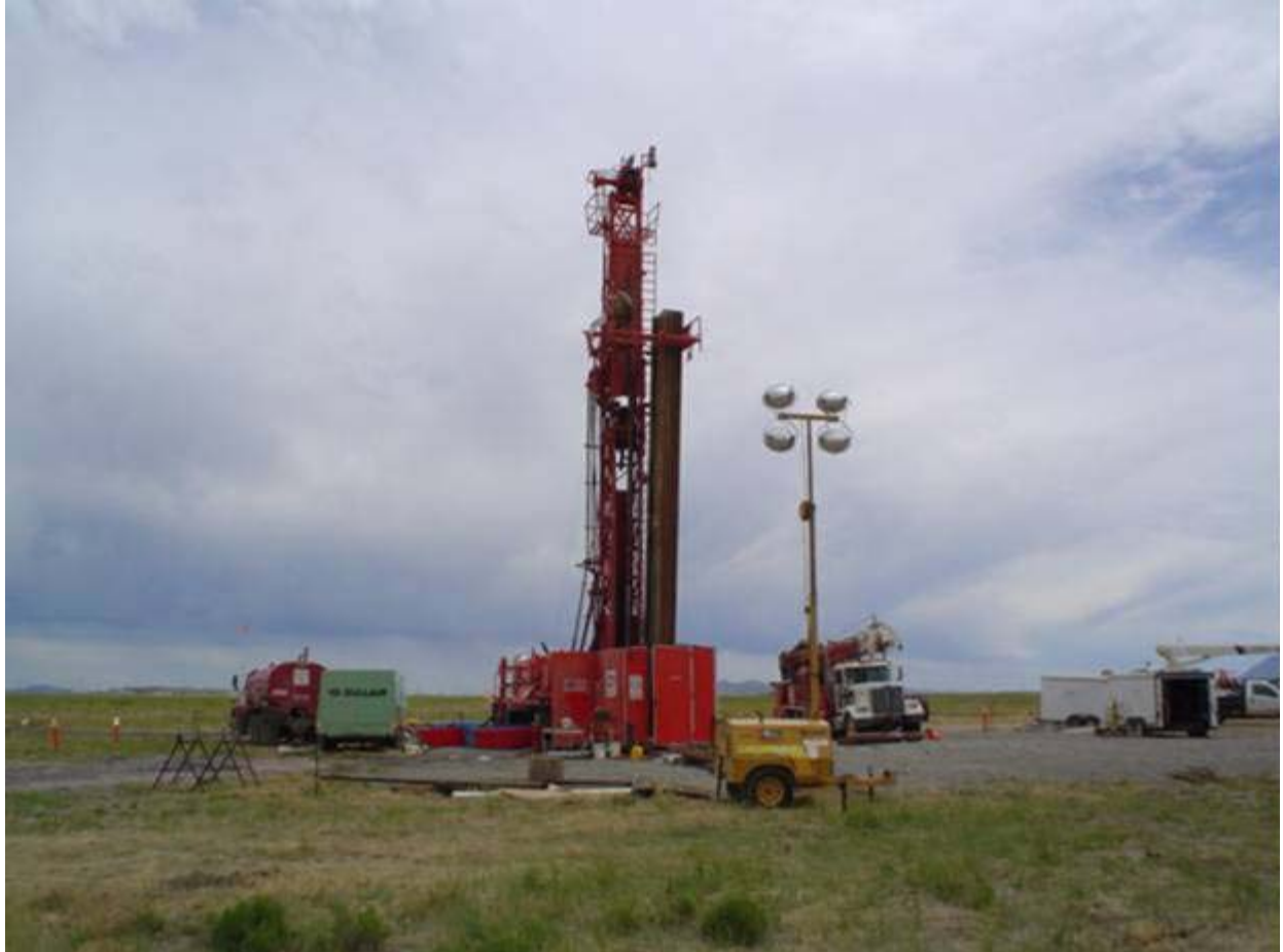
Figure D-2. Major's UDR-1500 drill/core rig and accessory equipment used for coring MIDDLE-2050A.
