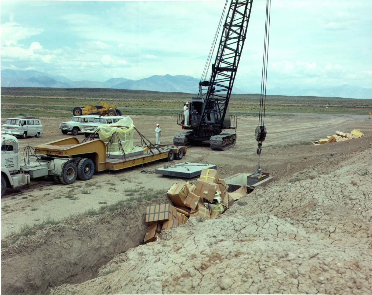
Figure 3-2. Waste contained in a waste insert being transferred from a shipping cask to a removable crib in Trench 55 in 1973 (photograph number 73-2345).
