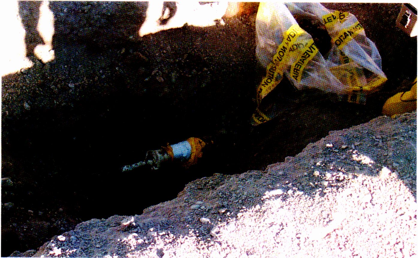
Figure 1: Picture of the south end of the carbon steel pipe where the proposed new site is located.
